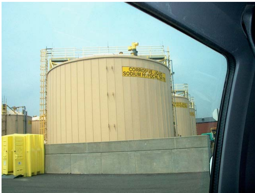
Deposits of sodium hypochlorite
