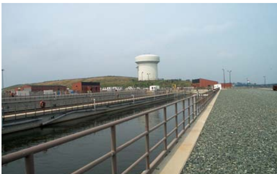
Clean water on its way to the minihydro before being sent to the outfall
